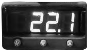
Temperature monitor/controller display and buttons.
