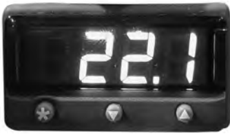
Temperature monitor/controller display and buttons.
