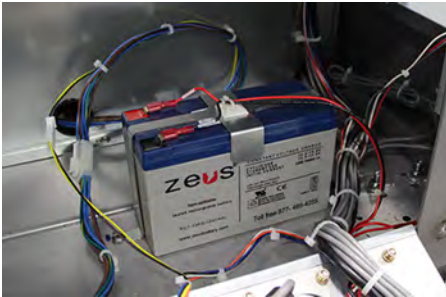
Monitoring system / Access control back-up battery
