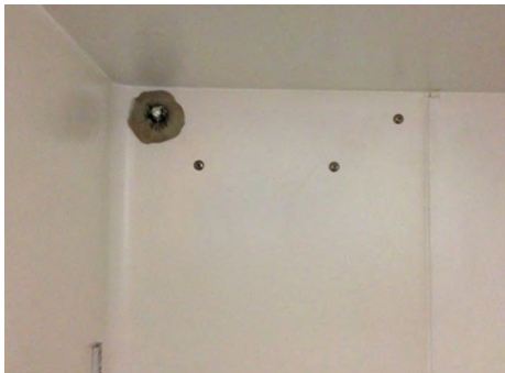
Threaded screw holes and distribution port for back-up refrigeration system installation
