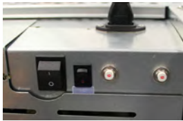
Figure 4: AC ON/OFF switch (left), monitoring system / Access Control backup battery ON/OFF switch (center), circuit breakers (230V systems only) (right).
