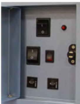
Figure 4: AC ON/OFF switch (top middle), i.C 3 monitoring / Access Control backup battery ON/OFF switch (center right), circuit breakers (bottom).
