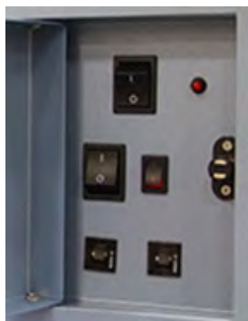
Figure 4: AC ON/OFF switch (top middle), i.C 3 monitoring / Access Control backup battery ON/OFF switch (center right), circuit breakers (bottom).
